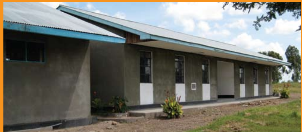
Kisangura Secondary – Girls' Dorm, unused due to lack of latrines (2009)
